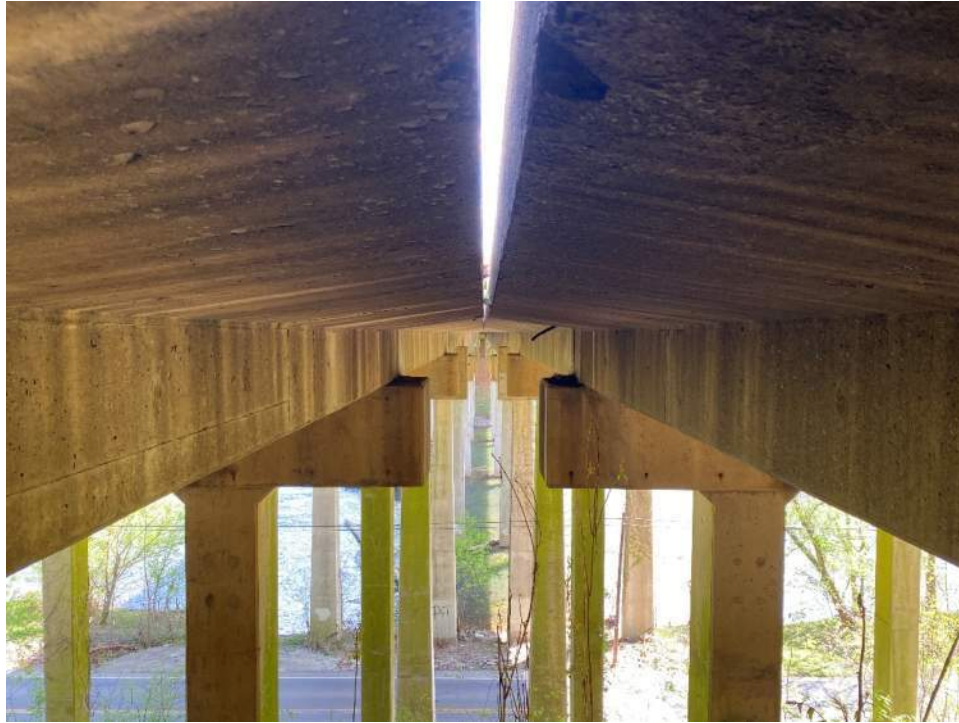
Gap between the two bridges
